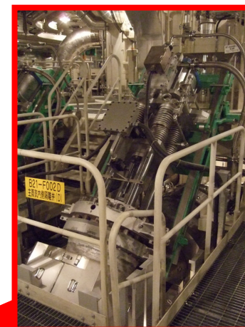
主蒸気隔離弁(8台)
